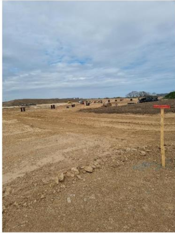
Photo 5 – Road formation with foul and surface manhole cylinders visible in the distance
