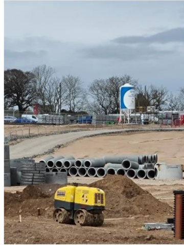
Photo 6 – View towards the compound area at the North-West corner of the site, with a mortar silo installed for underbuilding blockwork
