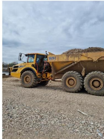
Photo 8 – One of the earth moving machines being used to help form required levels on site
